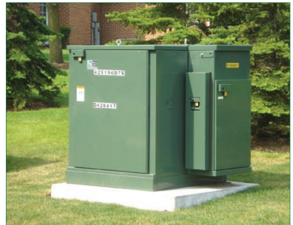
Pad-Mounted IntelliRupter PulseCloser integrates underground segments of a feeder with an IntelliTeam SG Automatic Restoration System.
