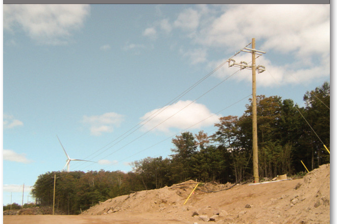
Prince 2 overhead collector system.
