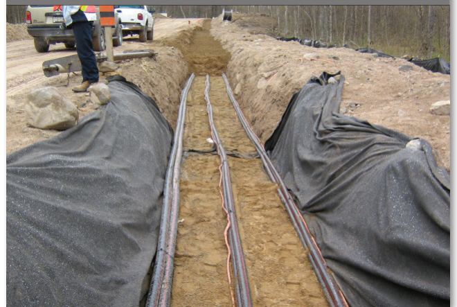
Prince 1 underground collector system.
