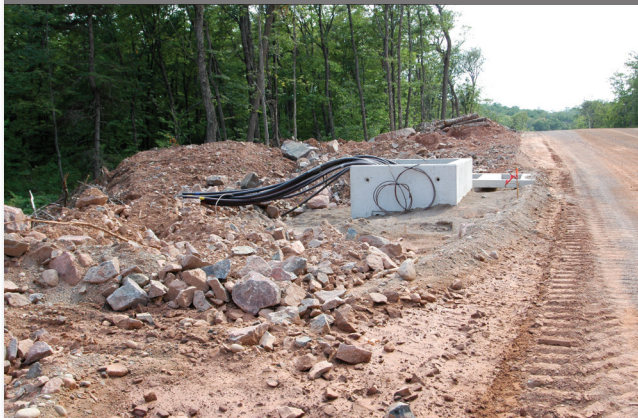
Pre-cast concrete vault for underground collector circuit isolation switch.
